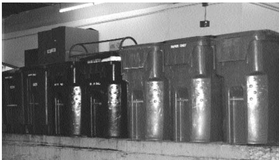
The hotel uses a refrigerator already installed on its loading dock to store food residuals so the hauler can make three weekly pick-ups versus daily collection.
